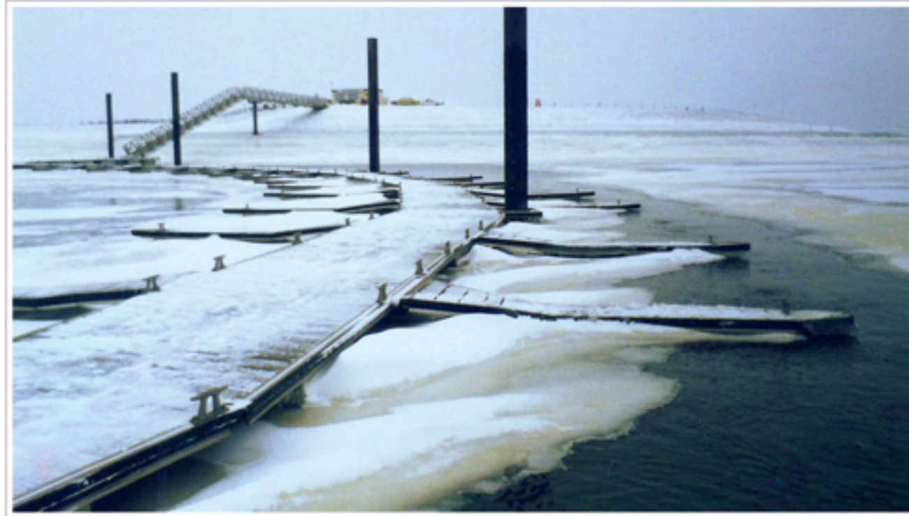
Ice Prevention Plant
